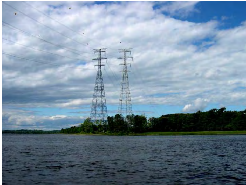
This is N of powerlines looking SW. Site was S. of lines.
